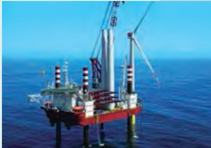
Offshore wind power facility installation project conducted by Seajacks International Ltd., which was acquired in 2012 (U.K.)
