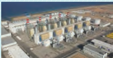
Sur Combined Cycle Power Plant (Oman)
