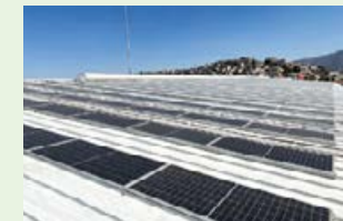
Decentralized power generation business (Mexico – Rooftop solar PV system)
