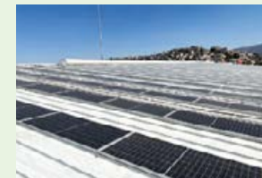
Decentralized power generation business (Mexico – Rooftop solar PV system)
