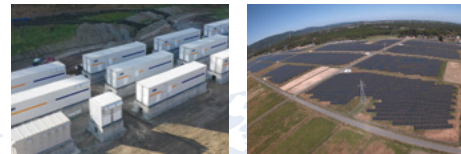
Energy Storage Systems Batteries
