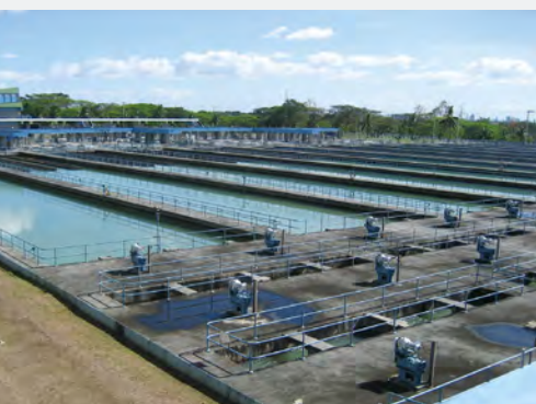
Site of water and wastewater services business of Maynilad Water Services, Inc. (Philippines)
