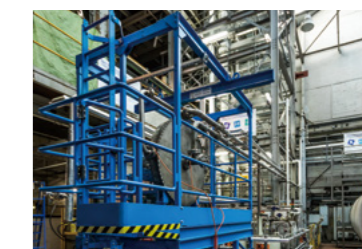
Next-generation carbon capture facility (CycloneCC) by U.K.-based Carbon Clean Solutions Ltd.
